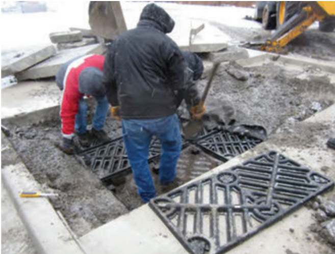
Manual removal of two decks, unscrewed and set aside for future re-installation.
