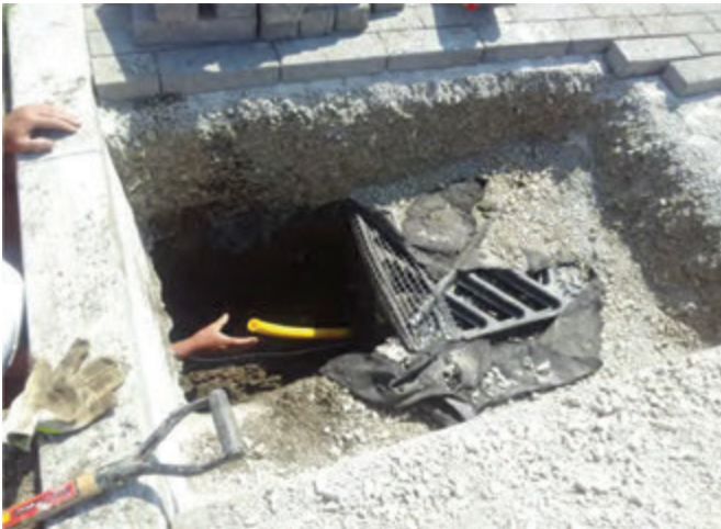
End of lateral at building end.
