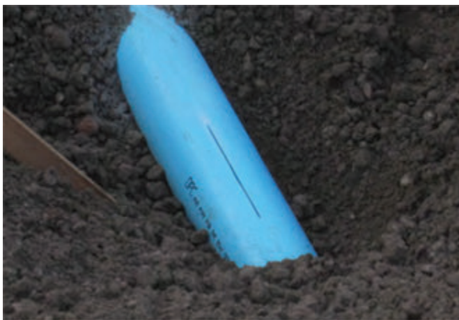
Water pipe cut.
