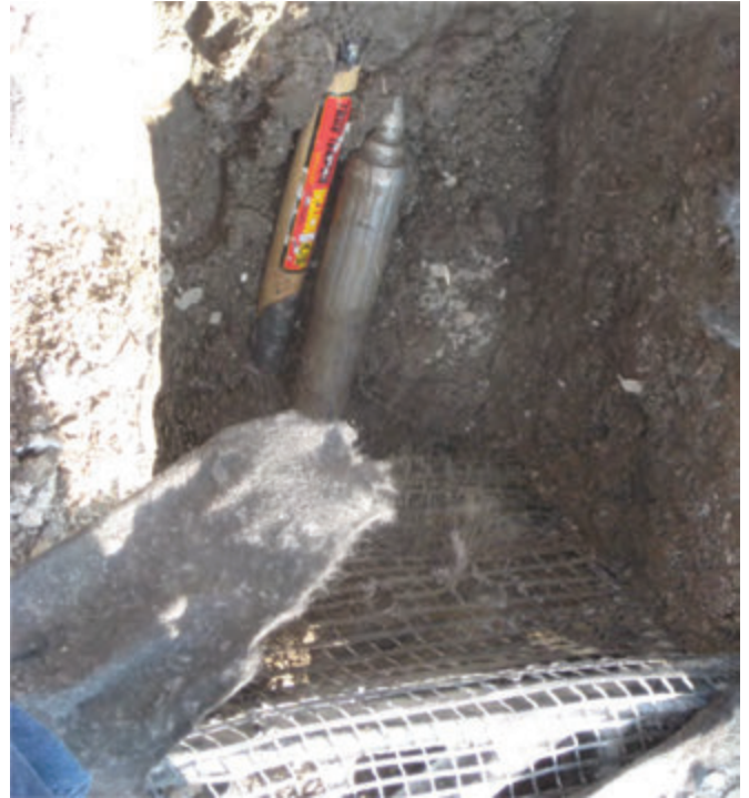
Torpedo emerges through growing medium and cell decks on the imaginary building side.
